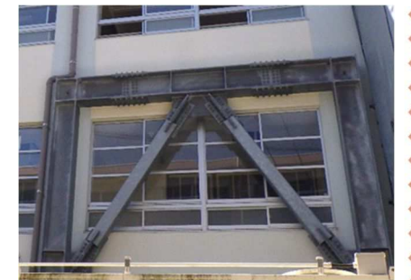
★耐震補強部材★
